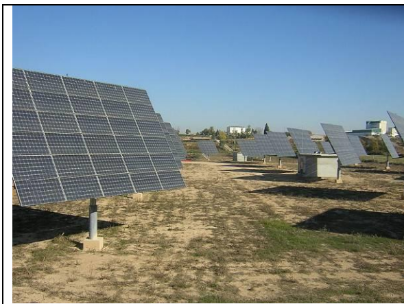
Figure 19: Example of solar arrays 12
