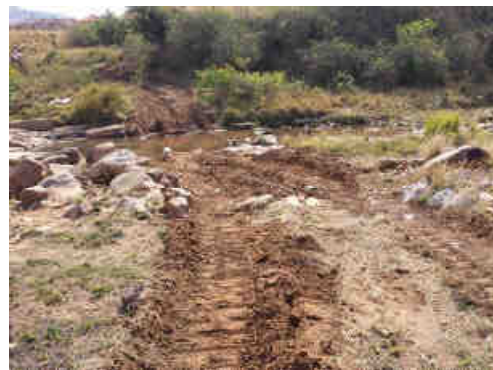
Photo 6: View of the crossing point for the preferred route (option 1) taken from the right bank to the south of the crossing. The crossing point has been recently disturbed upstream by heavy construction vehicles involved with maintaining an access road.
