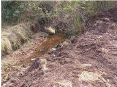
Photo 9: Riparian vegetation clearing and infilling of the tributary stream channel R03 associated with the construction of a new access road.
