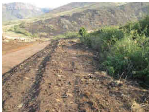
Photo 11: Newly constructed access road adjacent riparian zone of stream channel R03 with dense alien thicket.
