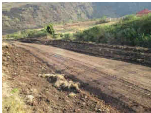
Photo 12: Another view of the newly constructed access road running along the edge of riparian zone R03.
