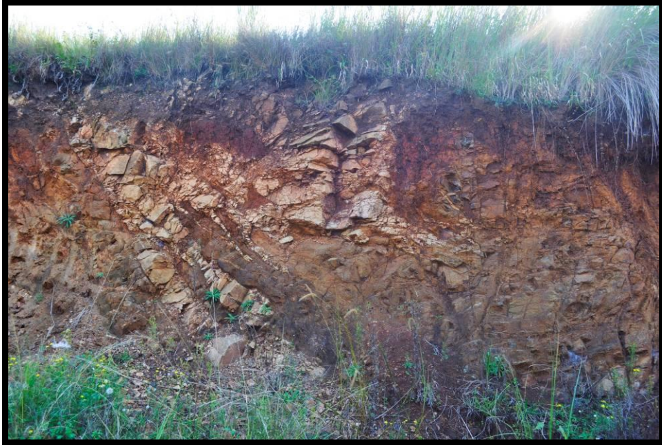
Figure7. The majority of the hillslopes in which the proposed Ntashana access road is situated on a shallow Orthic A layer with an underlying hard lithocutanic B horizon typical of the Glenrosa Form. The shallow soil layer is prone to erosion especially along the perennial and non-perennial drainage lines.
