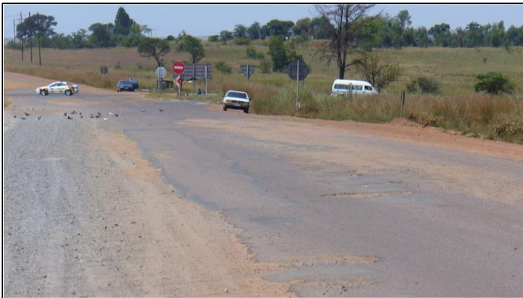
PHOTO 3: POTHoles ON THE ROAD TO ZITHOBENI INFORMAL SETTLEMENT - NOTE THE CARS DRIVING ON THE SHOULDER OF THE ROAD IN ORDER TO AVOID POTHoles
