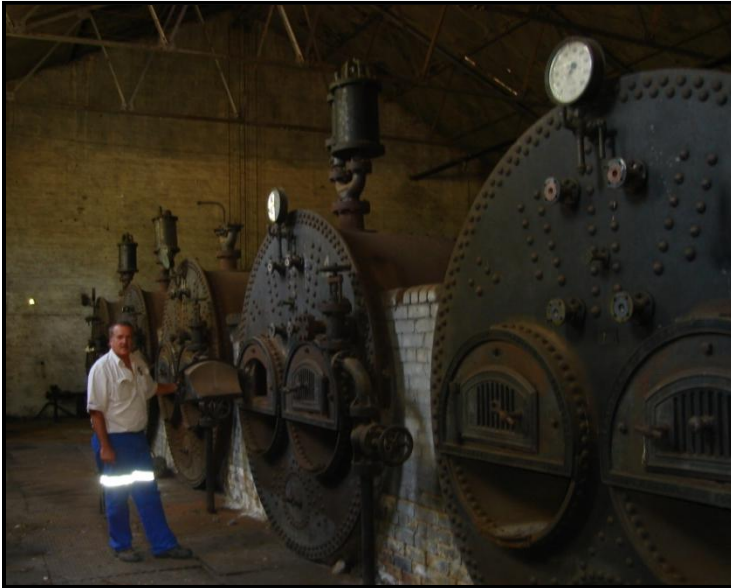
PHOTO 36: STEAM BOILERS AT WILGERIVIER PUMPSTATION
