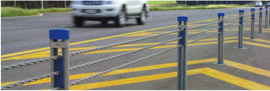
Photo 11.7.2: Wire rope barrier (Photo – http://www.armcorps.co.za )
