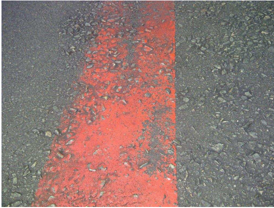
Photo 11.7.11: Solvent based road marking paint trial for Rea Vaya, photographed in 2011, three years after application in 2008 (Photo – L de Beer, GIBB, 2011)
